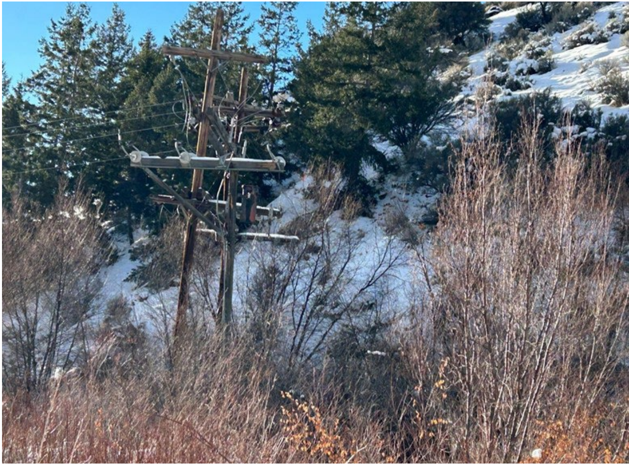
Figure 5.5. Power Line to Site by 360 Portal Source: Photo by AMPL, 2025
