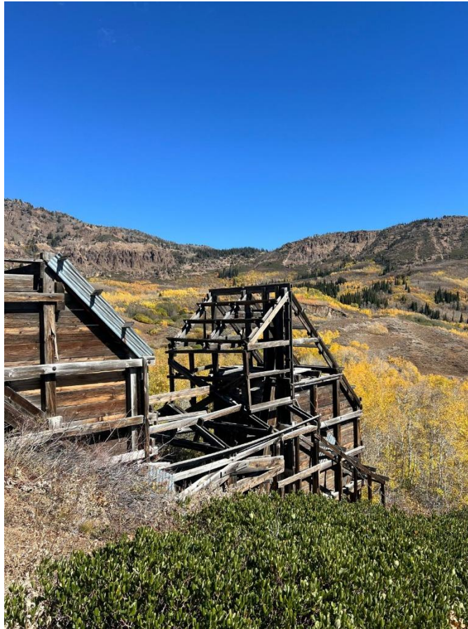
Figure 2: Infrastructure from past production at the Mission Cross Mine which is located on a single third party claim within the newly acquired White Star Property
